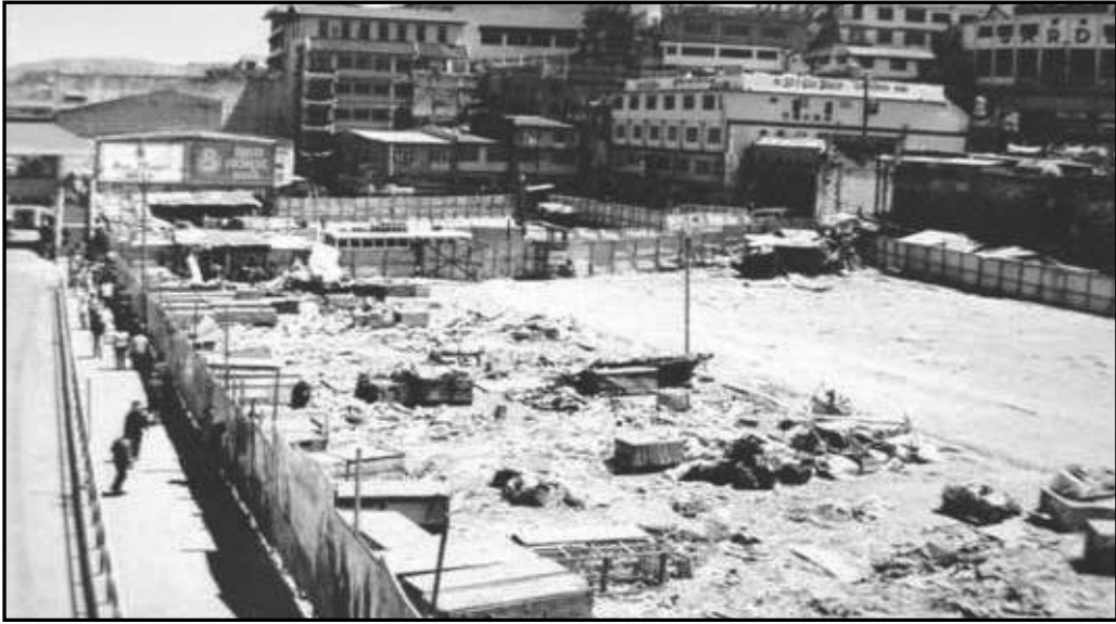
Figure 10. Ongoing construction of Baguio Center Mall ( from a photograph at the Kagitingan Barangay office ).
